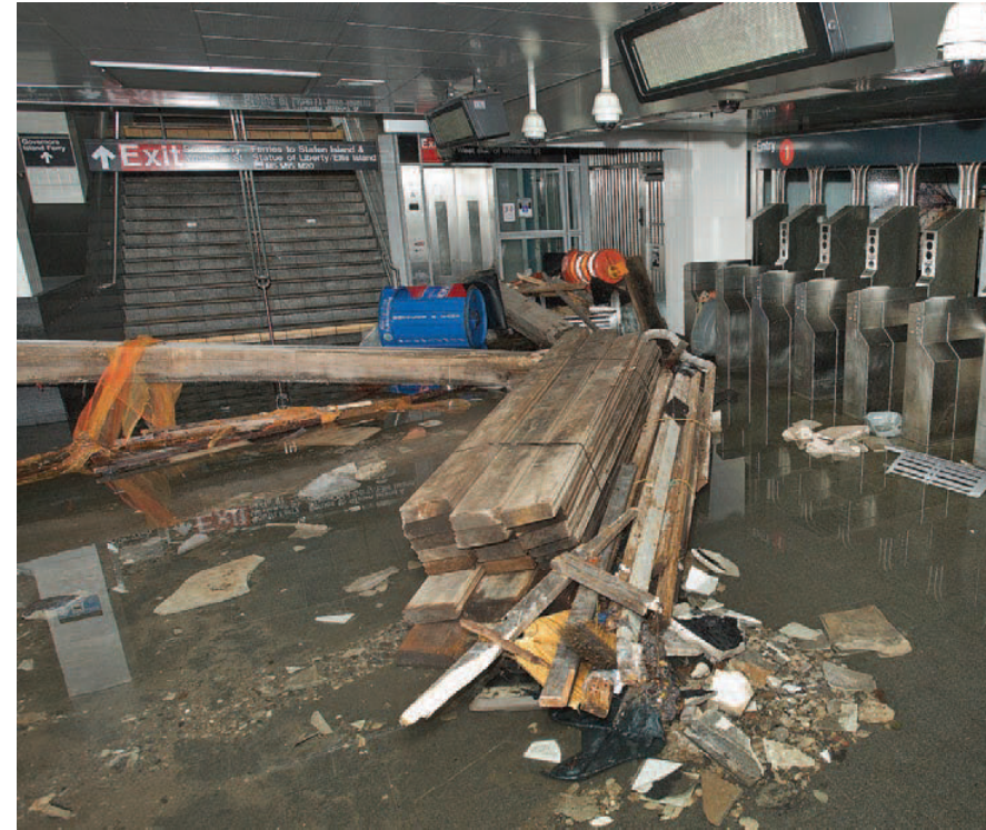
South Ferry Station in Lower Manhattan flooded to the mezzanine level after Hurricane Sandy (Photo Credit: MTA)
